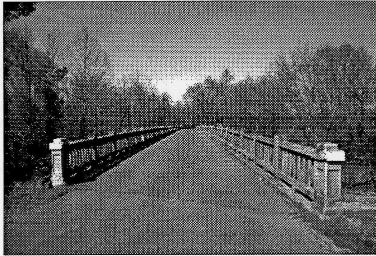
Figure D-13: This T-beam bridge, which is located near Armuchee in Floyd County, Georgia was built in 1924, and has been determined to be individually eligible for listing in the National Register of Historic Places (photograph by author).
